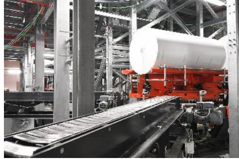
Automatic Reel Storage 10.000 T
