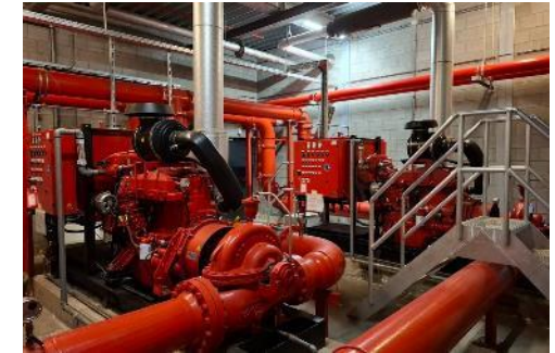
Fire Station Engines
